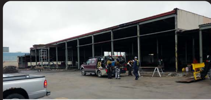
The building with the front removed before installation of a new front.
