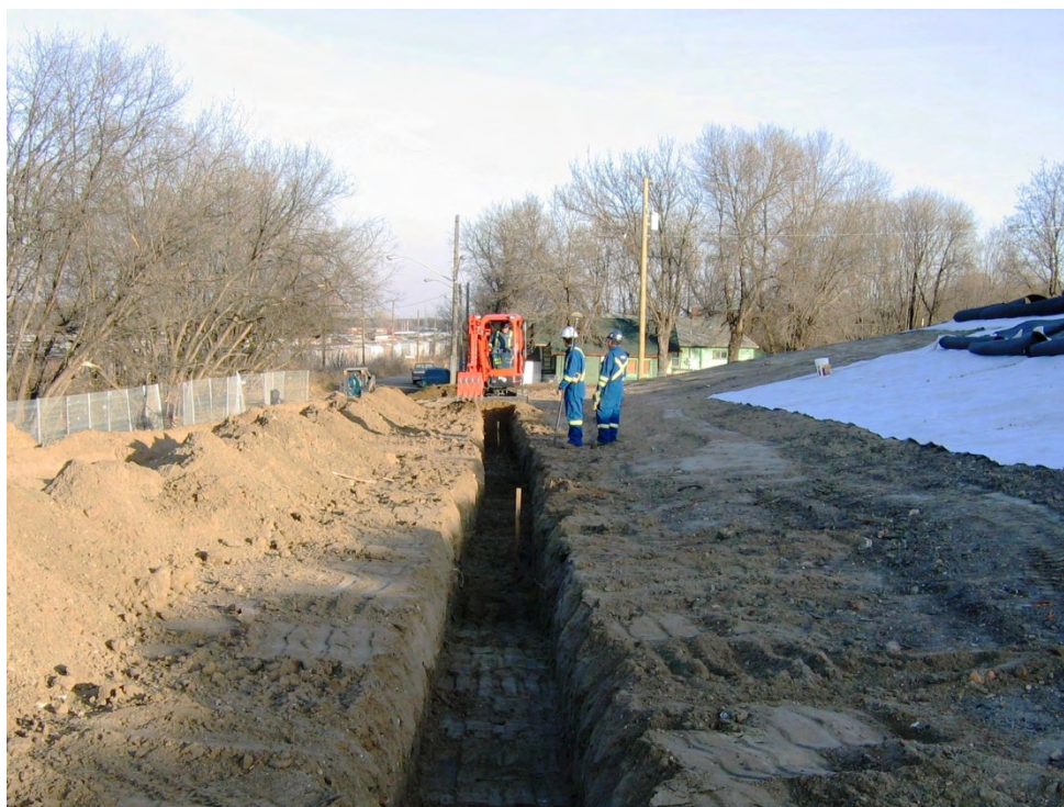
Photograph 14. Drainage trench construction along north side of engineered cap. Photograph facing east. (October 2008)
