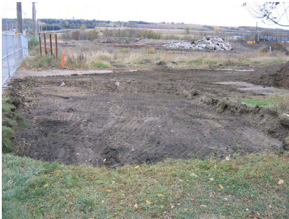
Photograph 7. Surface soil excavation on west side of Site. Photograph facing north. (October 2008)
