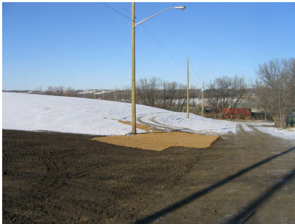
Photograph 17. Completed east side of engineered cap, including walking path. Photograph facing north. (November 2008)
