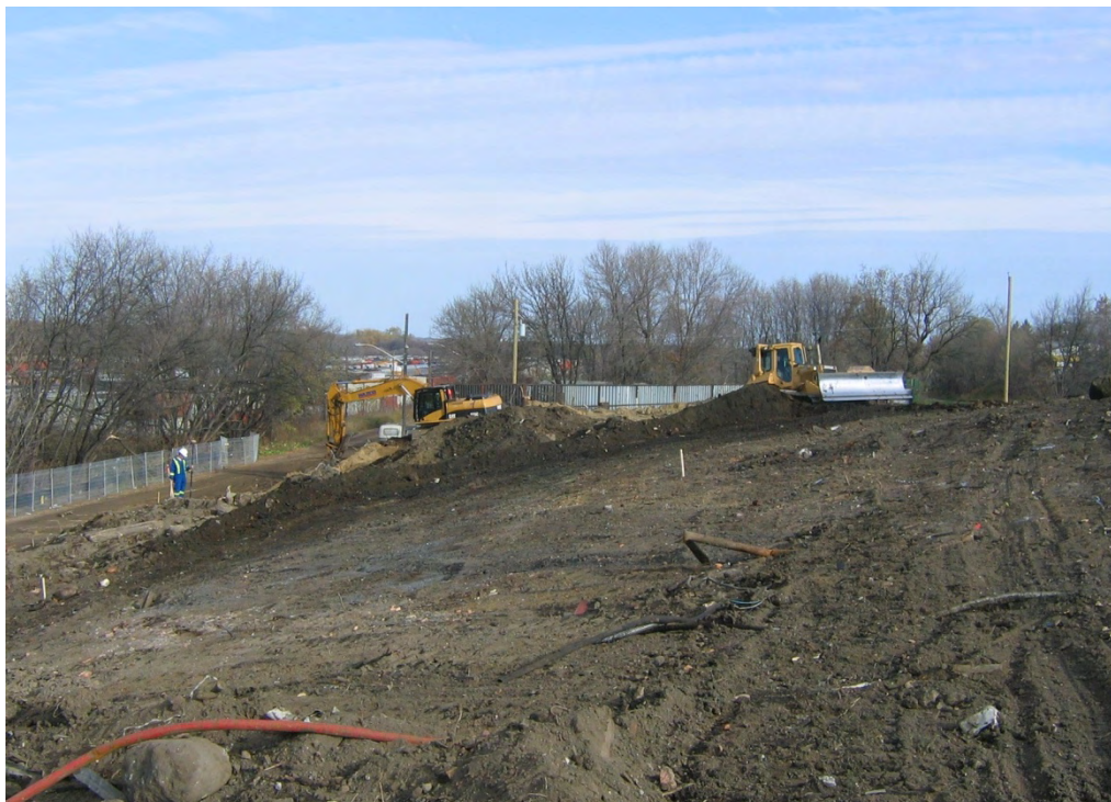
Photograph 10. Grading of soil prior to placement of engineered cap. Photograph facing east. (October 2008)
