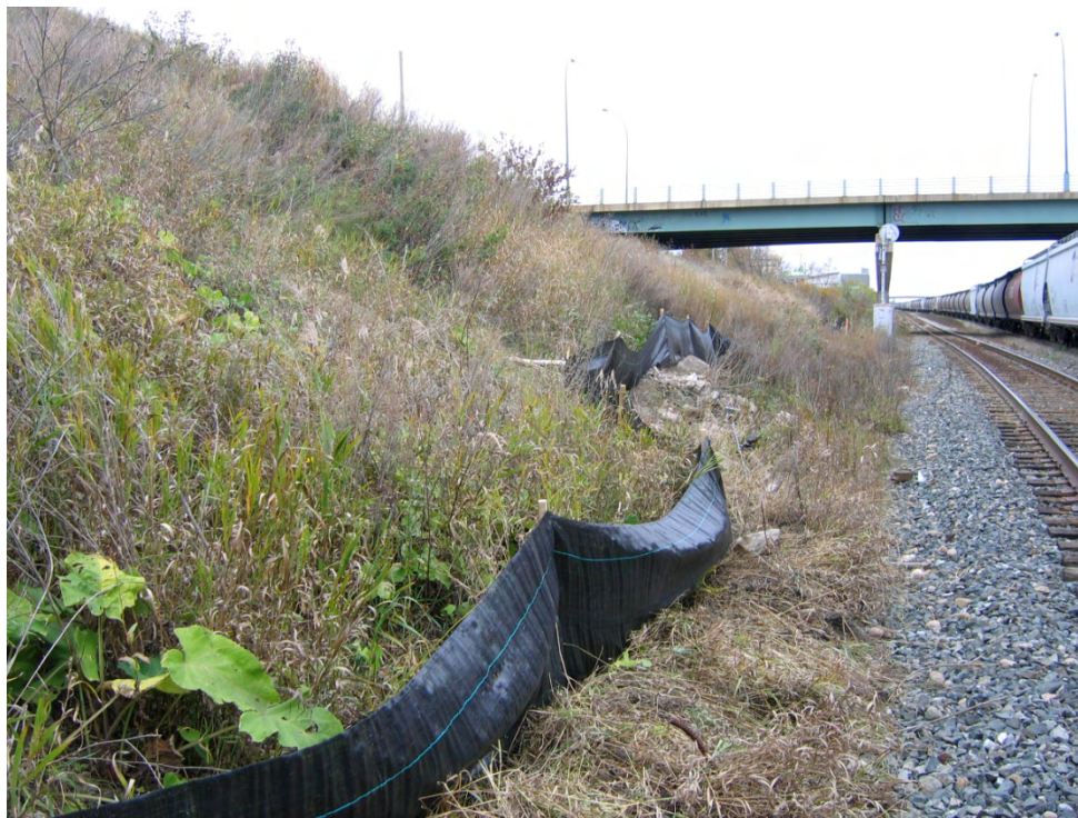
Photograph 3. Silt fence installed north of Pacific Avenue prior to construction activities. Photograph facing west. (September 2008)
